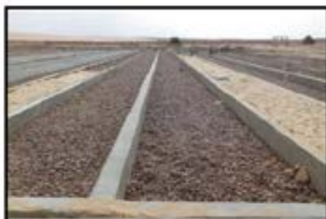
Figure 11. channels in the GBH CW at Sinai. Photo Credit: Abdel-Shafy et al., 2022. https://doi.org/10.1007/978-3-031-03600-2_5
