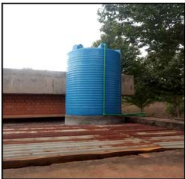
FIGURE 10 : An tank above « the AMPHI building » with the volumes : 2500 liters
