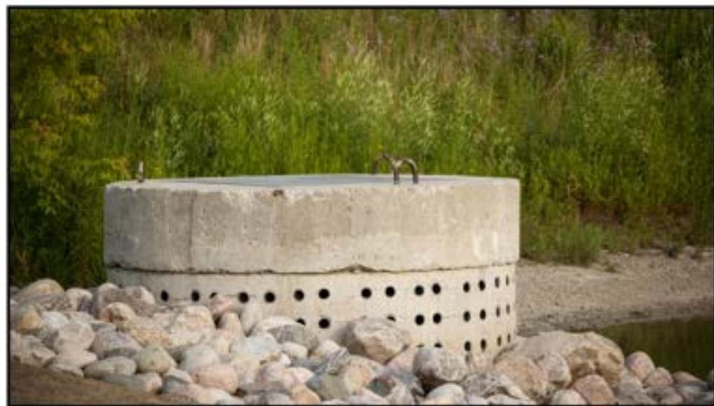
Figure 3: Stormwater Management Infrastructure, Perforated Concrete Pipe Photo Credit: Brian Guest/Canva Pro
