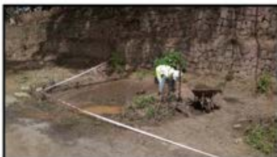
Figure 2: The obstructed manhole
