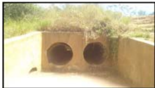
Figure 4: Stormwater Runoff being routed to the Rice Fields (Zone I) Photo Credit: FINARCH
