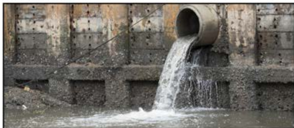
Figure 4: Storm Drain Outlet - the volume is not small. Photo Credit: Nuttanun/Canva Pro
