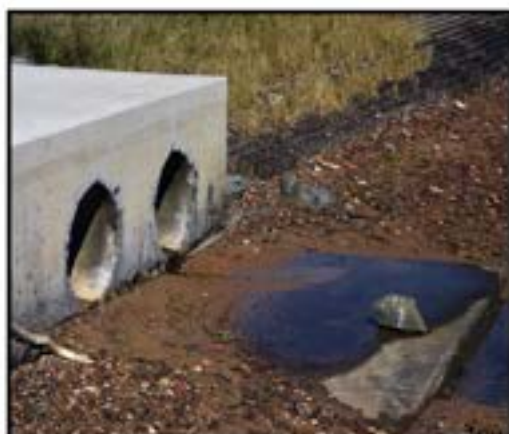
Figure 5: Stormwater Outlet Pipes - Typical rerouting of the storm flood Photo Credit: Scott Kenneth Brodie/Canva Pro
