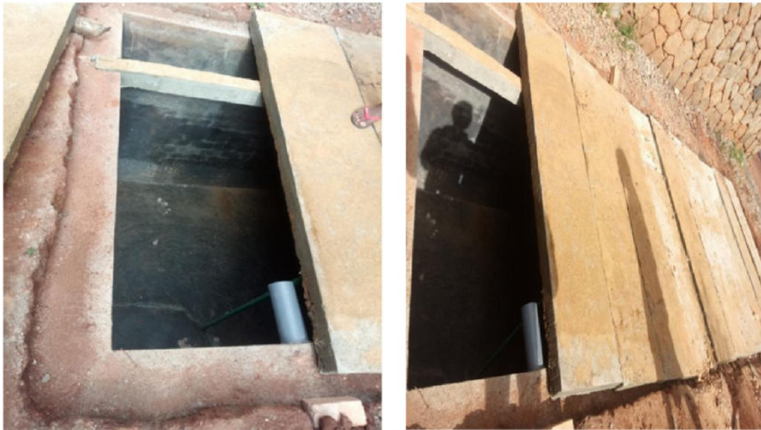
FIGURE 7 cistern underground « near of the economics department »
