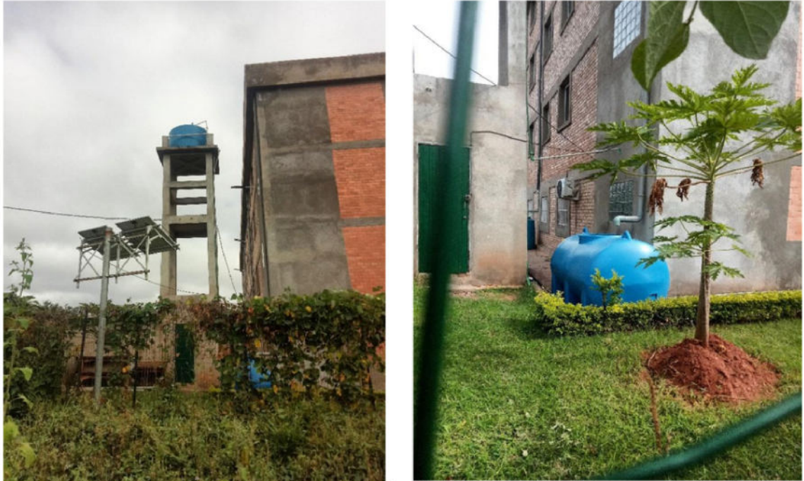
FIGURE 5 : An areal blue tank and the horizontal tank in the building of the « Madagascar Institute for Vaccine »
